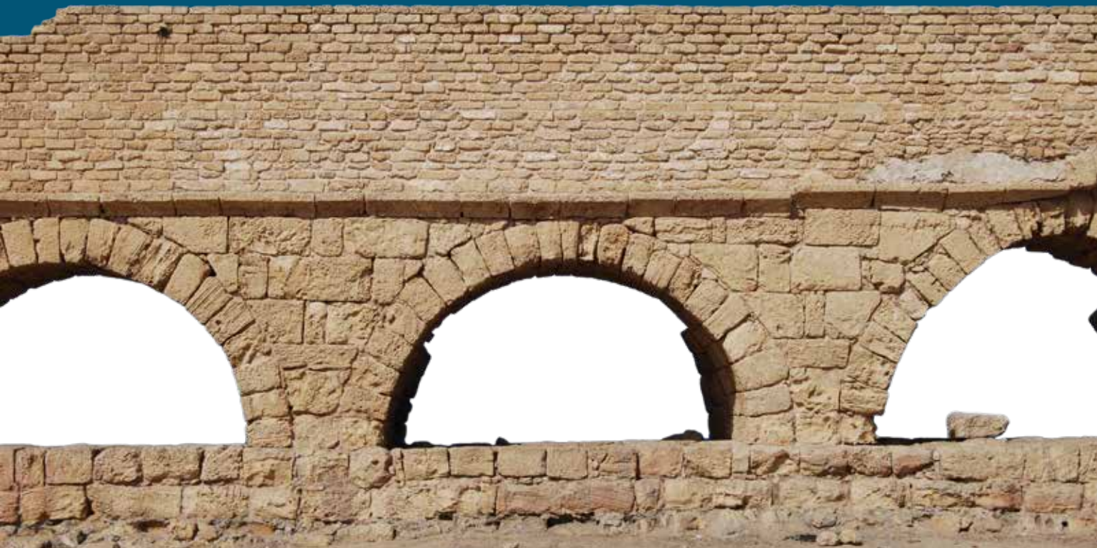
The aqueduct Herod built at Caesarea-Maritima brought water from the Shuni spring, south of Mount Carmel, about six miles NE of the city.
